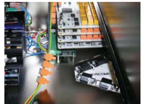
Detail of YAV switching boards and serial bus interface mounted in the back of a VPC Receiver
